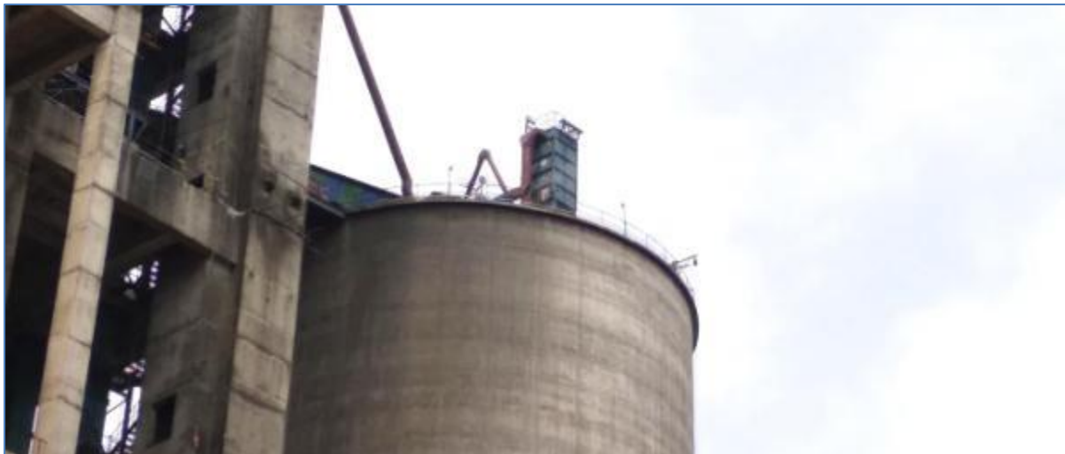
Bag Filters at Blending silo Top
