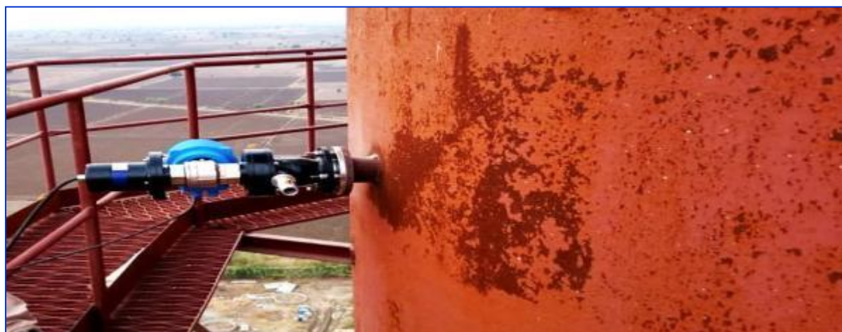
PM CEMS for Clinker Cooler ESP Stack
