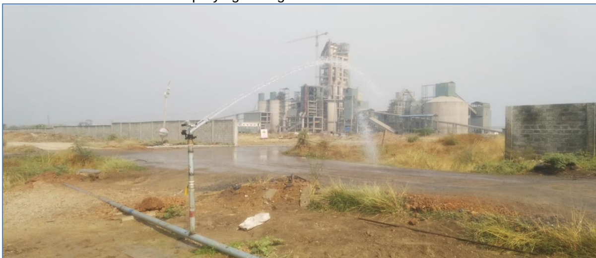
Water spraying mechanical sprinklers on internal roads
