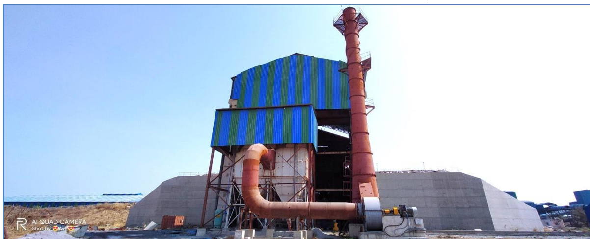
Bag Filter at Limestone Primary Crusher
